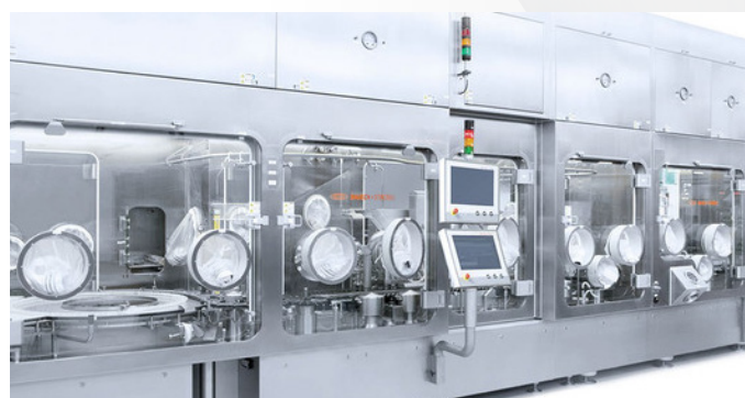
Vial filling and stoppering machine within an isolator enclosure. The air-handling capability of the isolator is integrated into the isolator unit. In contrast to the RABS doors, the doors of the isolator are thicker and are fully sealed, typically by inflatable gaskets, against the door frames of the isolator. The image also shows two glove ports on each door, which allow the operator to make manual interventions without opening the isolator doors. Image courtesy of Bausch+Ströbel. Used with permission.
